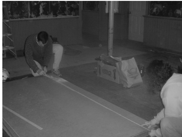
Steve and his wife, Sue, measure one of the hardboards before cutting. The couple mounted all 140 feet of the future blackboards in one day. After the special black paint is applied, wood trim will be added to frame each section of the boards.
