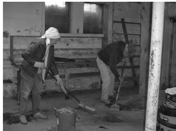
Judy and Harlan Corrie remove old tile from floor of basement room in 1889 school.
