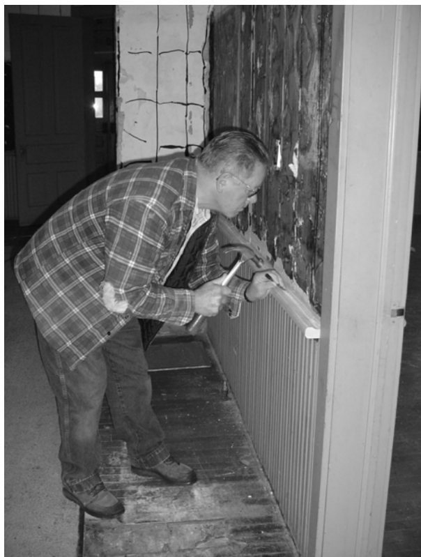
Cedarville's Darrell Baker replaces chalk holder beneath blackboard in first floor north room of 1889 school. He also repaired damaged floor boards and wainscoting.
